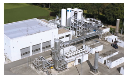
Power-to-Gas plant operated by kiwi AG in Werlte, Germany
