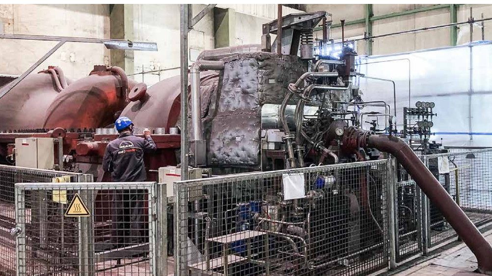
Original Siemens steam turbine from 1975 before replacement.
