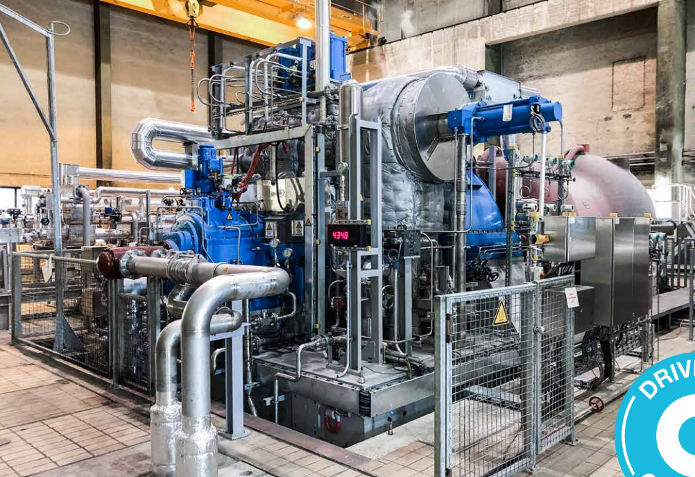
New MAN MST080 steam turbine integrated for optimal performance.
