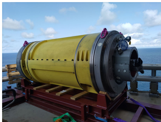
One of the three RB compressor bundles installed and commissioned by Everllence on Equinor's Troll A platform in the Norwegian North Sea. © Everllence
